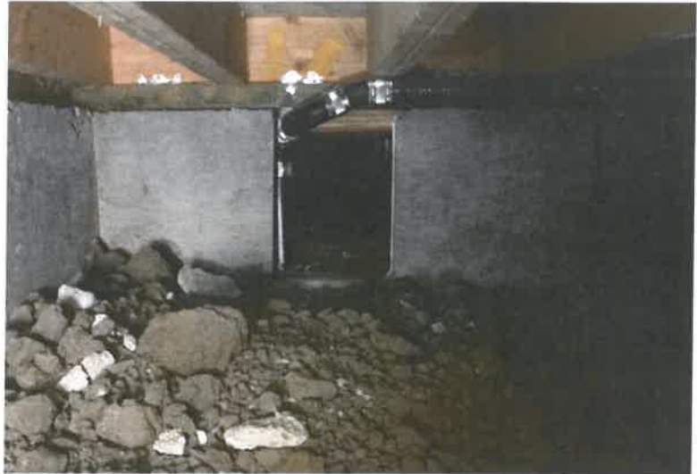
Photo 7: 07/13/18 Interior – Front of Home Vent that is Across from Outside-Back- Front Vent
