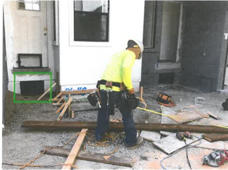
Photo 4: 04/17/18 Front of Home – Vent Under the Stairs. Before finished construction of Stairs.
