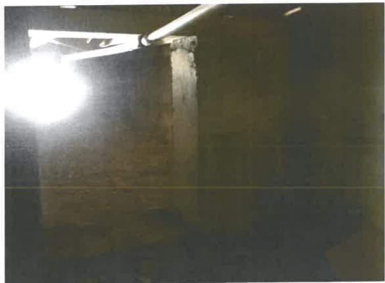
Photo 9: 07/13/18 Interior – Front Vent In between the Garage North Wall Vent And the front of home Vent under the stairs
